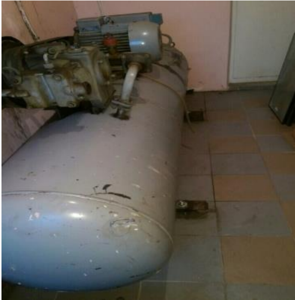
Fig. 6. General view of the compressor structure anchored to the acrylic composition
